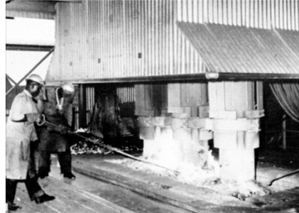
Three-in-line 3.5 MVA furnace, pioneered at Driehoek and transferred to Middelburg. In 1969, it was shown that round sub-arcs with electrodes in a triangle would be 50% more efficient, so they were changed.
