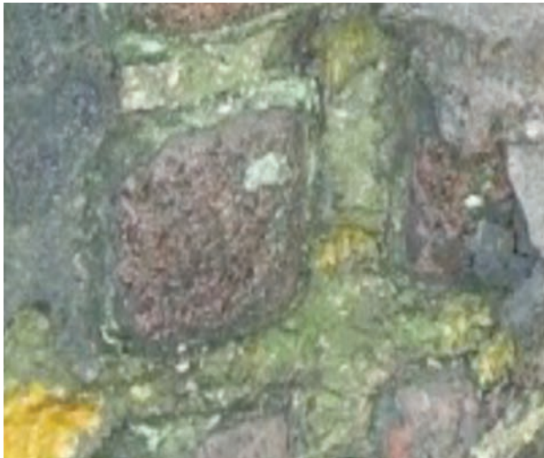
Figure 6—Typical corroded cooler – yellow elemental sulphur deposited on black copper sulfide corrosion product on copper. Grey covering is frozen slag accretion
