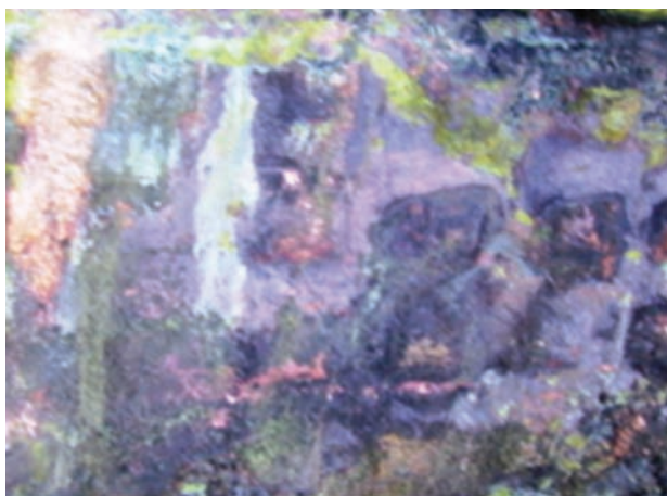
Figure 7—Severely corroded, unprotected copper block. Black copper sulphide pervasive. Increasing evidence of green copper hydroxy-chloride in close proximity to copper
