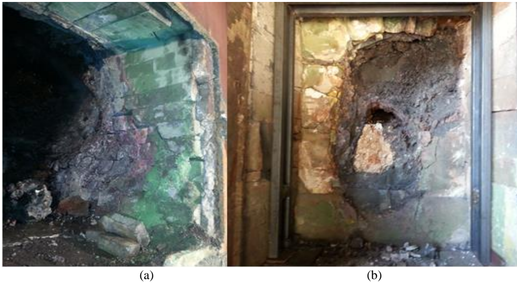
Figure 4 – (a) Tapping hole lining maintenance, Vargön Alloys AB ,Sweden (b) Tapping hole lining maintenance, Eti Krom Inc., Turkey
