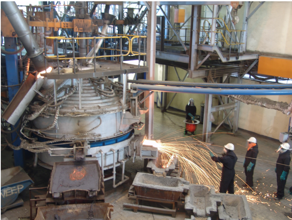
1.5 MW DC arc furnace at Mintek, 2007
