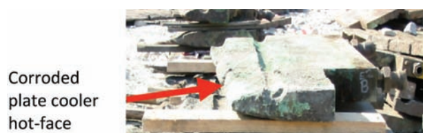
Figure 4—Severe upper plate cooler corrosion at Waterval Smelter. Note increased corrosion of upper plate cooler located in the furnace nearest the top of slag and concentrate interface
