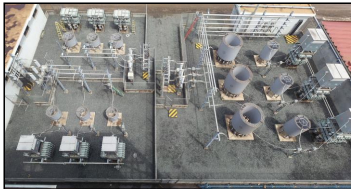
Figure 23: SVC at Case Study Location
